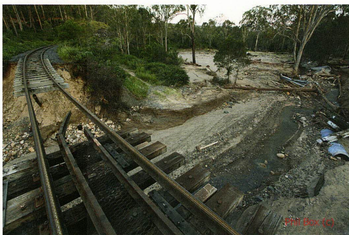
Floodwaters eroded the supports of this rail bridge in the Lockyer Valley
